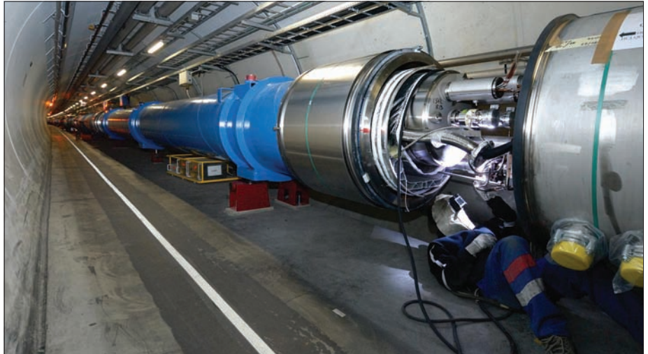
A welder at work on LHC sector 1-2. This is the last sector to be interconnected.
